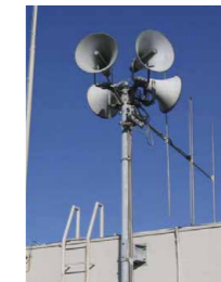
Emergency broadcast system Photo by Chiyoda City, Tokyo
