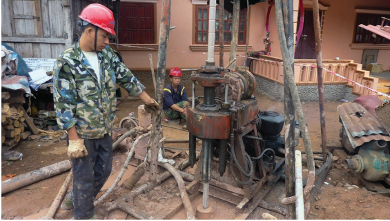
Chinese workers operating a drilling machine in preparation for building the railway linking China to Laos in Bopiat Village, Louang Namtha province, Laos, Hoang Dinh Nam/AFP/Getty Images, March 10, 2011
