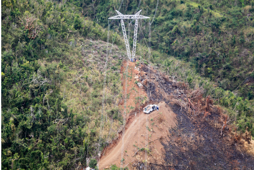
Transmission tower in the Montaña Area, Caguas, Puerto Rico. The power grid remains in fragile condition and much of the infrastructure is in hard-to-reach areas. Courtesy of the South Atlantic Division, US Army Corps of Engineers.
