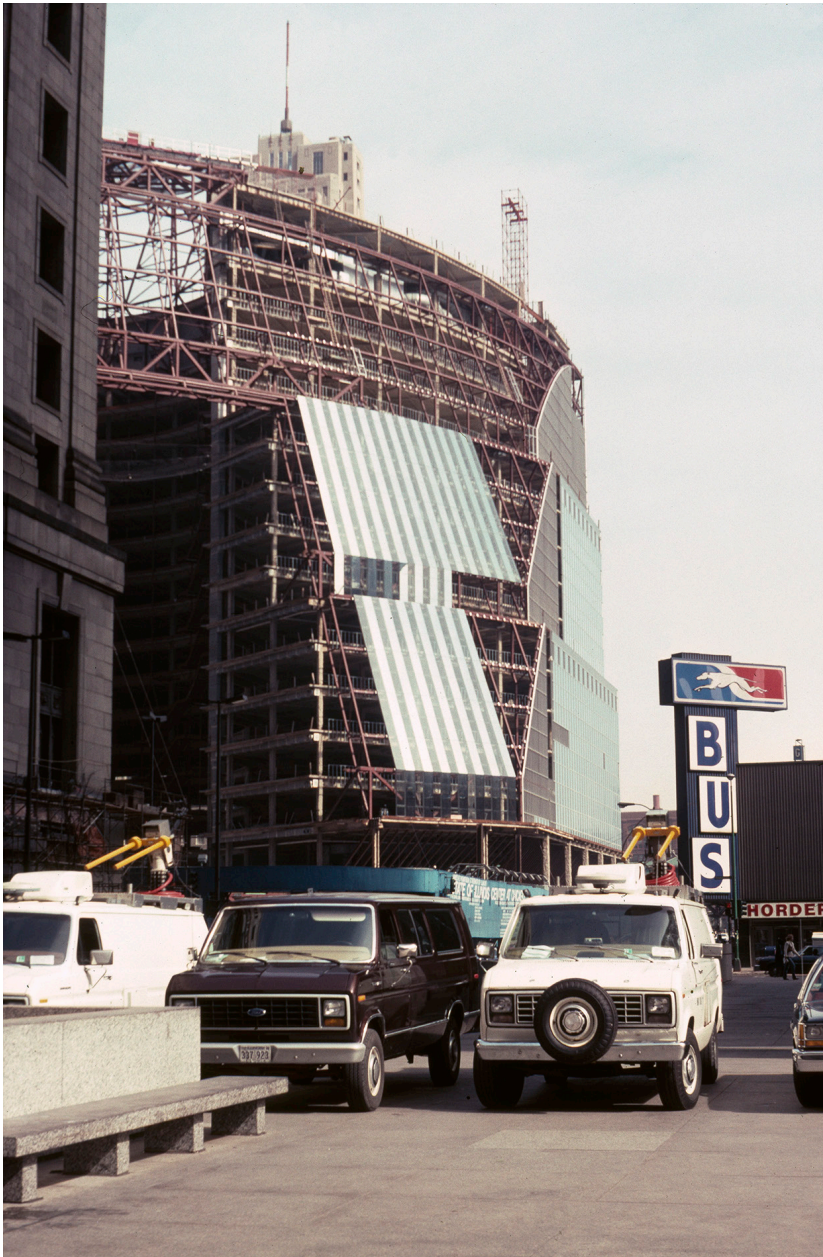
James R. Thompson Center, State of Illinois Center, under construction, 1983. Photograph by C. William Brubaker. Courtesy of C. William Brubaker Collection, bru003_05_jF, University of Illinois at Chicago Library.
