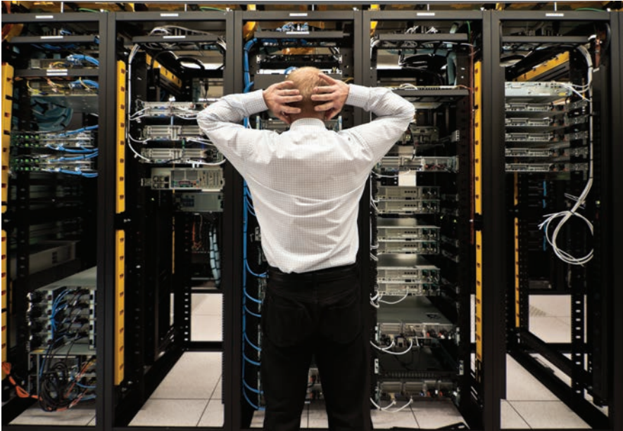
Figure 10-1 Racks of Equipment
