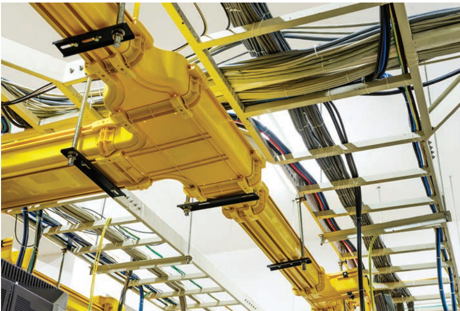
Figure 10-10 Overhead Cable Tray
