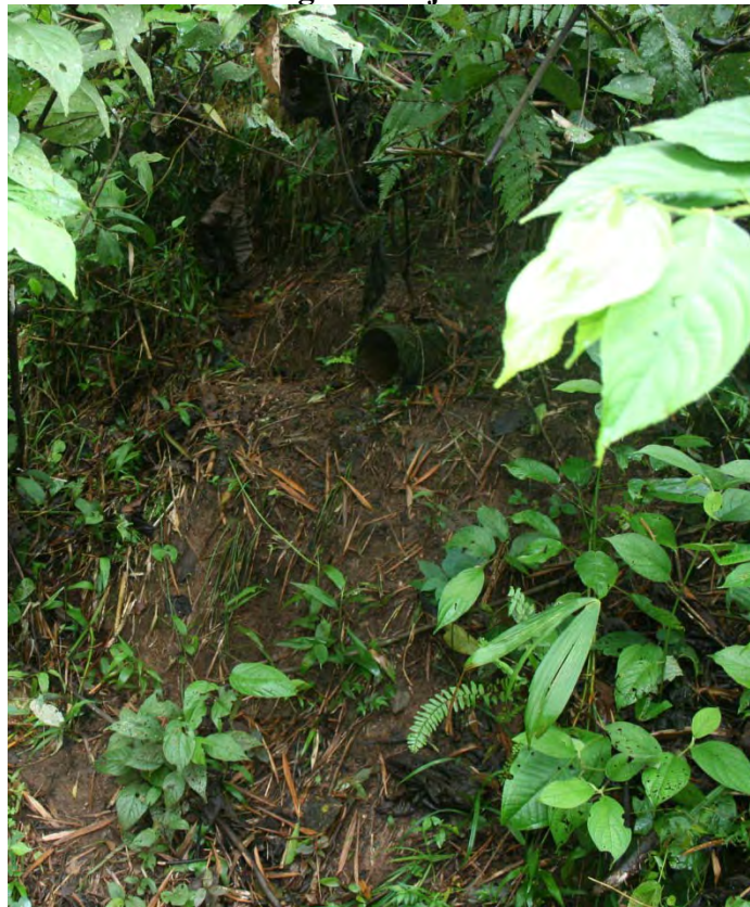
Figure II-5 Drainage pipe in side of Pit 3. The contaminated stream is immediately below the pipe.
