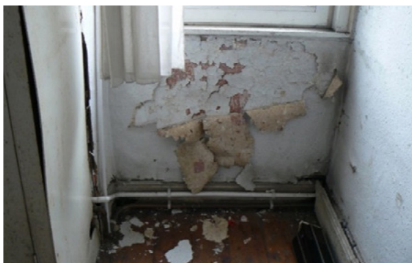
Figure 4: Category 1 dampness and mould growth
