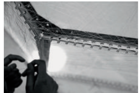
Fig. 10: Knotting of vertex connections of non-woven silk patches on temporary aluminium scaffolding structure.
