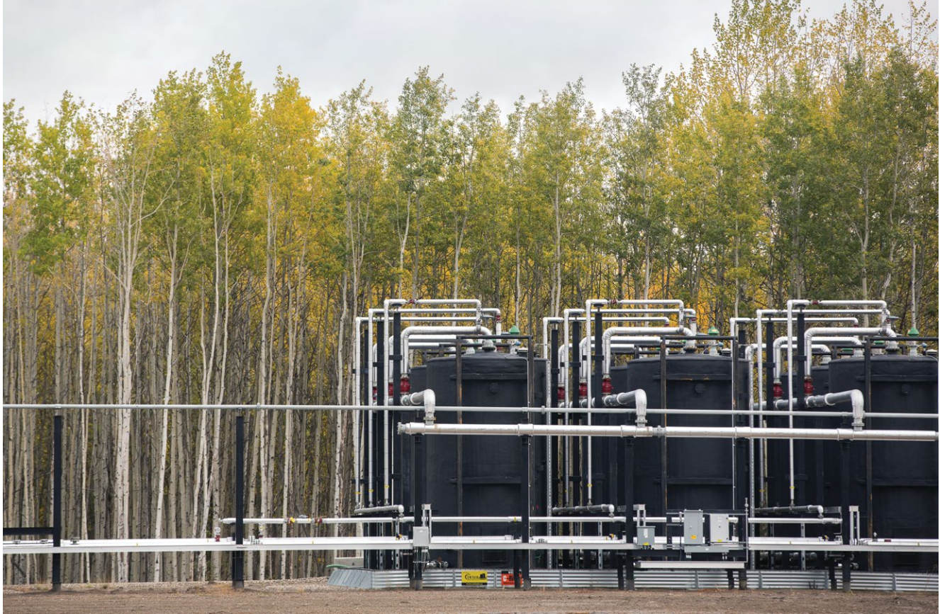
Compression dehydration facility, Montney, British Columbia
