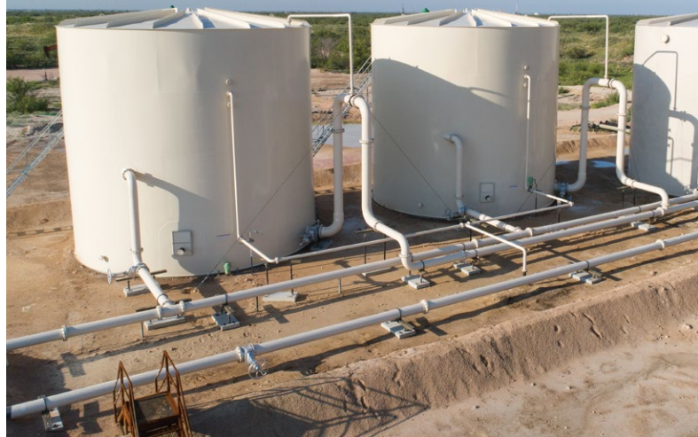
Tubb McKnight Water Station, Permian, Texas
