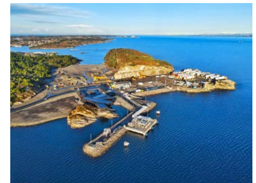
The Northern Lights CO 2 receiving, storage and pumping terminal, now under construction in Øygarden, (Norway).
