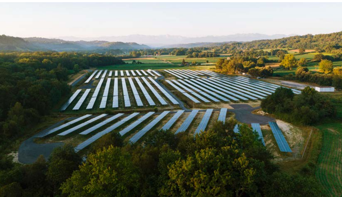
The Monein solar power plant in Pyrénées-Atlantiques (France), developed by TotalEnergies Renewables.
