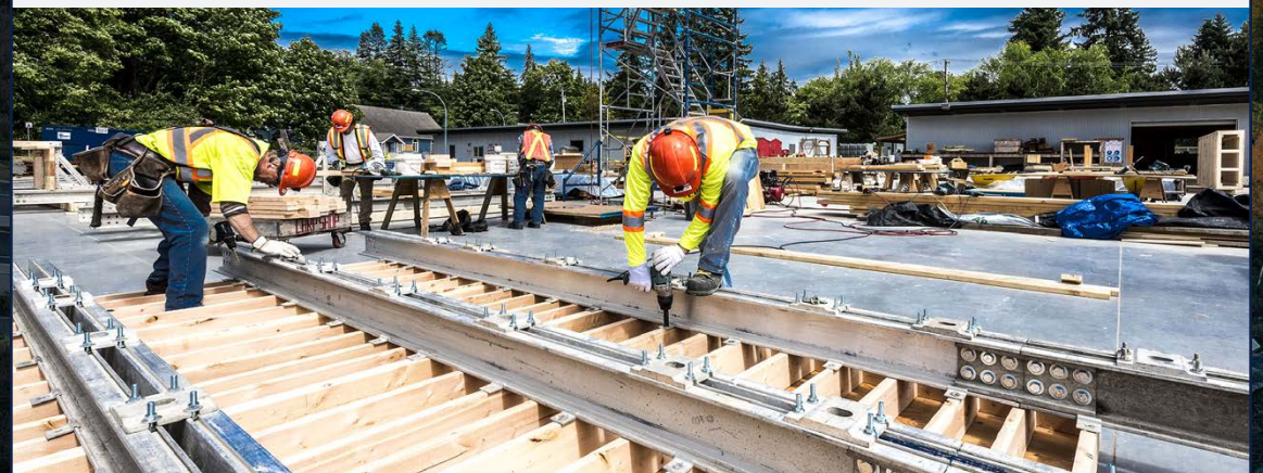
John Hart Dam Seismic Upgrade Project, British Columbia. Aecon leads the consortium in upgrading earth stabilization for stronger seismic resilience.
