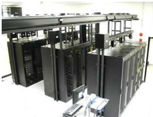
Figure 23 Example of a modular busway system.
