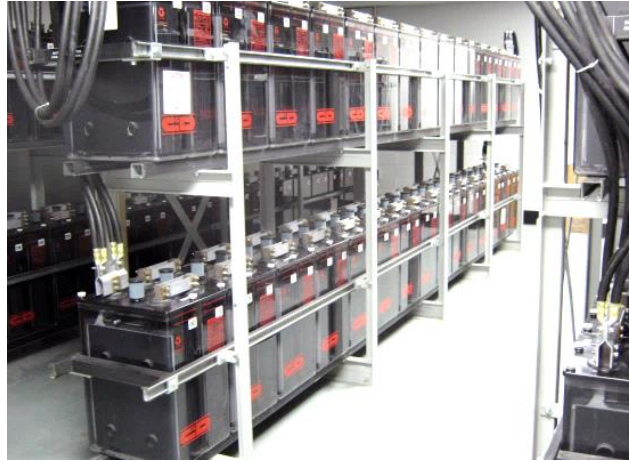
Figure 15 Data center UPS battery room with flooded cell type batteries.
