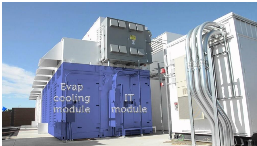
Figure 5 Air-side economized modular data center with evaporative cooling module.
