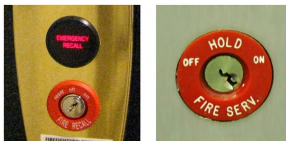
Figure 3. Elevator fire service key switches.
