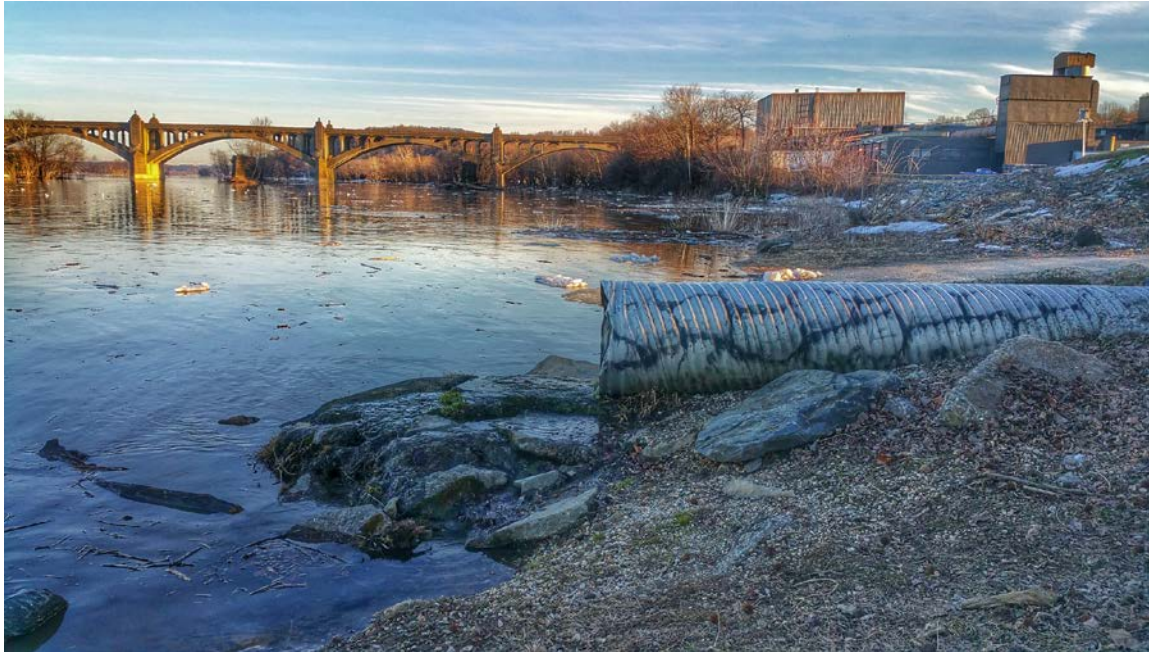
This photo highlights the importance of maintaining Wrightsville's stormwater infrastructure which flows directly into the Susquehanna River; Photo credit – E. Reed
