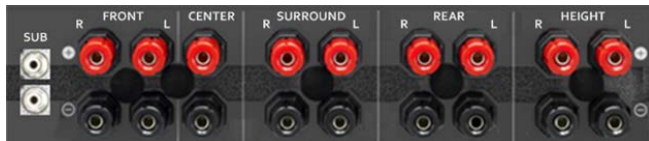
Figure 7: Rear panel of AVR; the height speaker connections are at right.
