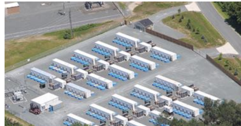
Beacon Power 20MW
