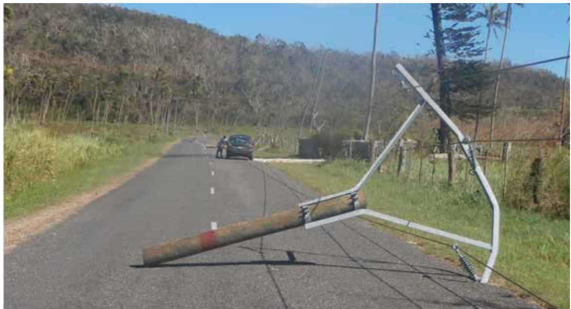
Damaged power lines in Efate. Source: Government of Vanuatu.
