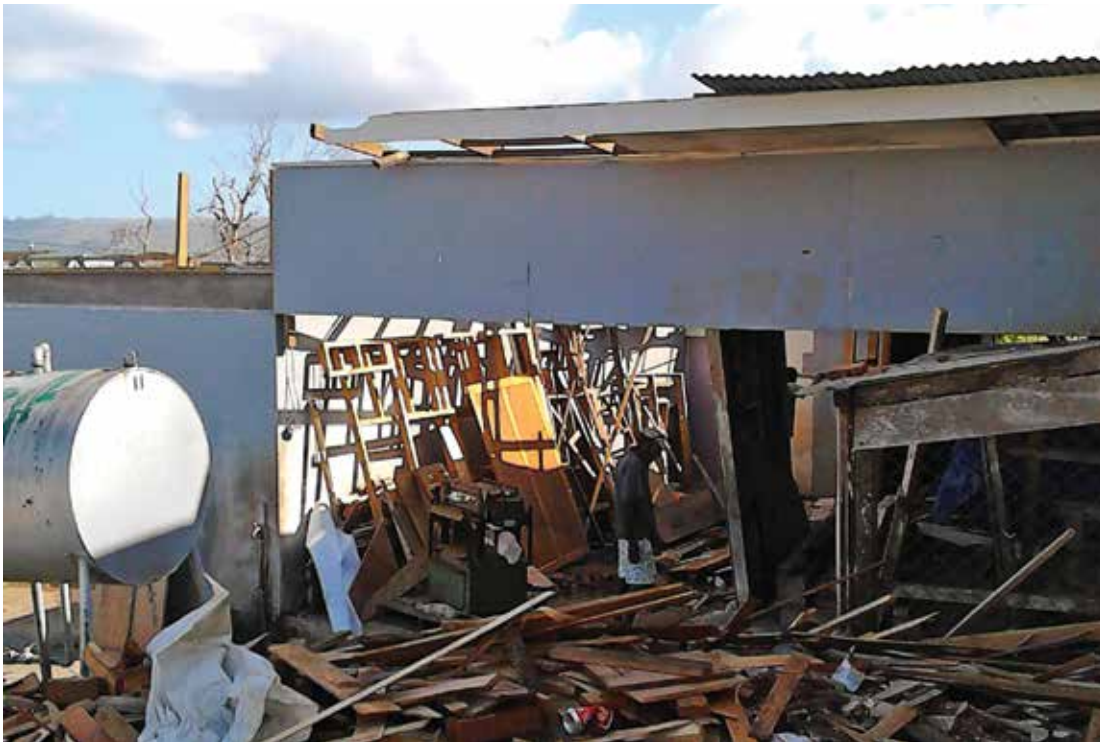
Damage to North Efate Timber, a factory in Port Vila, Shefa Province. © Lazarus Aising, Vanuatu Dept. of Industry.
