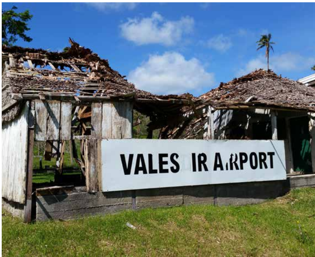
Cyclone damage to outer island domestic terminal in Epi. © Michael Bonte-Grapentin, World Bank Group.
