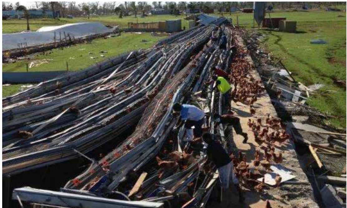
Damage to poultry shade at Chicko Farm, Efate Island in Shefa Province. © Jimmy Rantes, Vanuatu Dept. of Industry.
