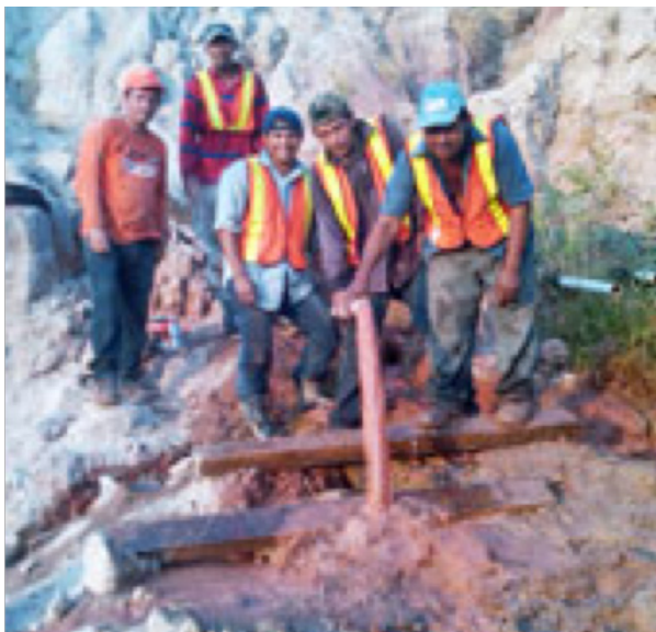
Photo 4.3: Drained Subsurface Water at a Sliding Road Mountainside Slope
