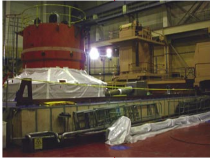
After removal of nuclear fuel, reactor vessel is shielded for decommissioning work
