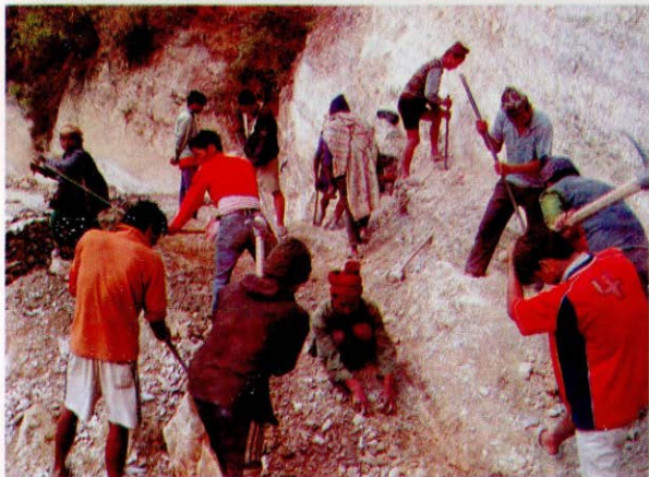
The construction of Shaheed Marg is going on with the people's and PLA's support
