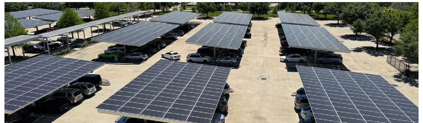
The TGS Houston Operational Headquarters landmark solar energy parking canopy in Houston, Texas. Consisting of 1,700 modules, the installation is projected to boast an annual output of 929,034-kilowatt hours of energy – creating a unique approach to achieving the Company’s net-zero targets.
