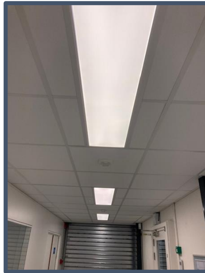
Figure 4: LED lighting with motion detector in the production area
