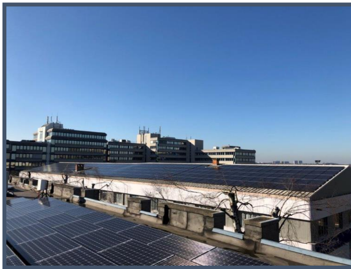
Figure 5: Solar panels installed on the roof of our HQ in Brussels
